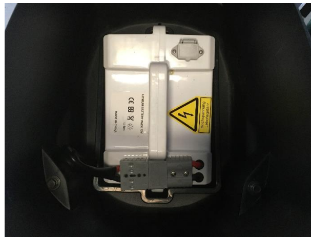
Discharge plug connected
