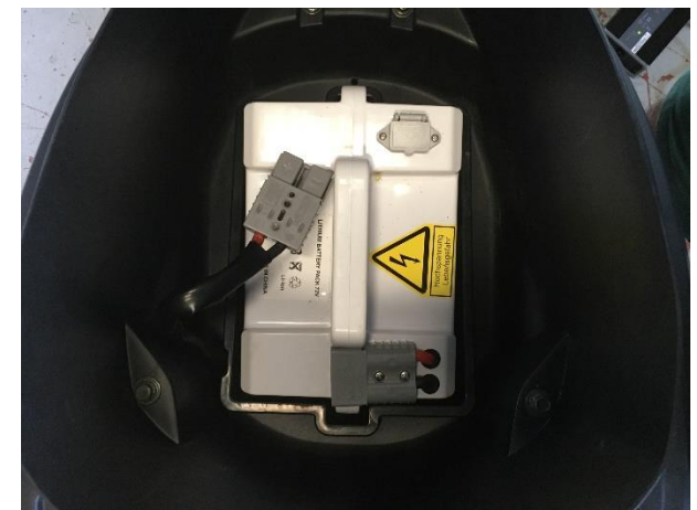
Discharge plug disconnected
